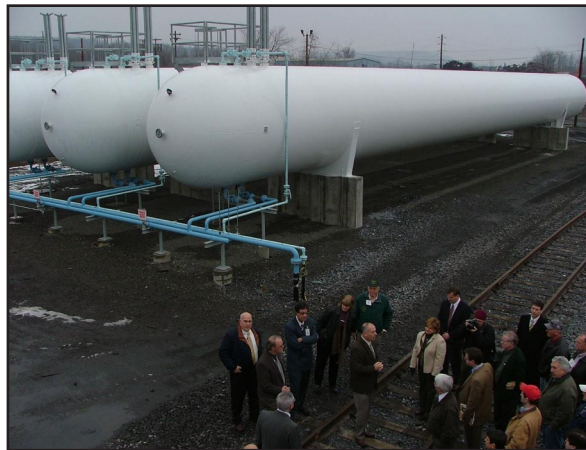
With UGI's storage tanks in the background, the group gathered for the ribbon-cutting.
